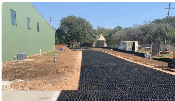
Photos: Recent photos of construction are shown on the Creed Ford III Therapeutic Riding Ranch at Marbridge.
